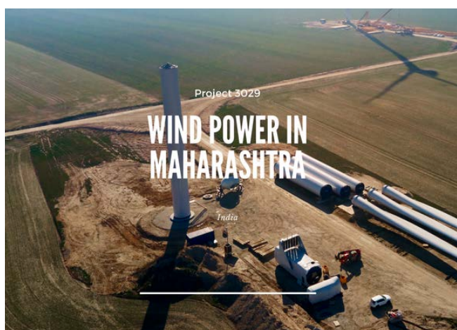
Project 3029: Wind Power in Maharashtra
